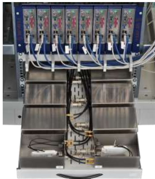
Fig. 3: Arrangement of 8 RF Guards on a single rack shelf
